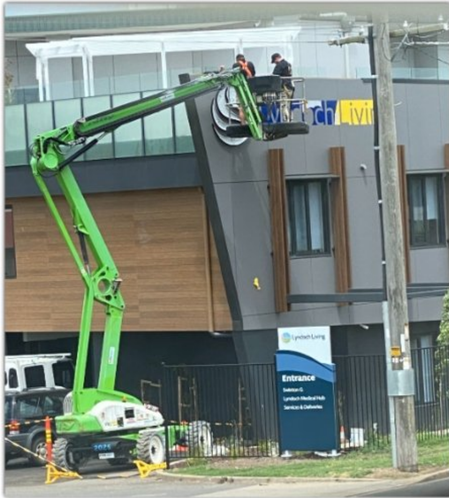
The Cassign team installing new signage today on the Swinton Wing expansion at Lyndoch Living.
